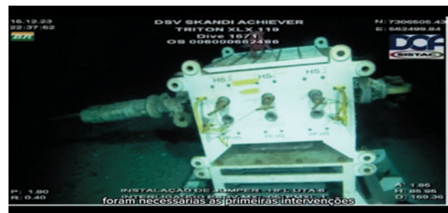
Figura 1: ESDV ( Emergency Shut Down Valve ).
